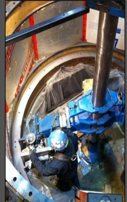
Field Service & Testing
